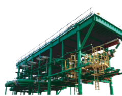
Pipe Process Module
