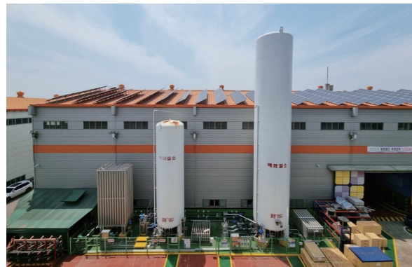
Test Facility (LN2 Tanks)
